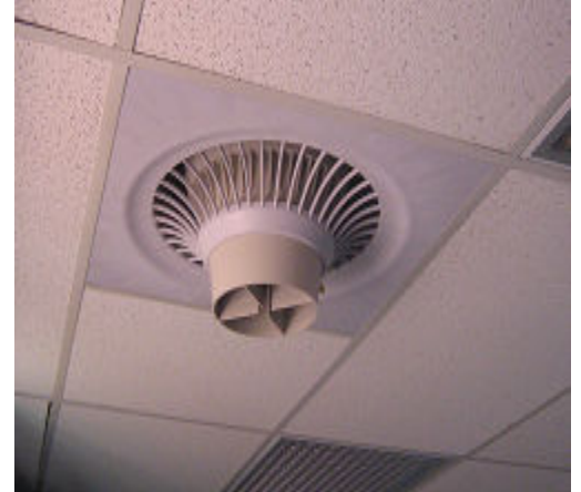
Suspended Ceiling Kit Installed with AIRIUS Unit in Place
